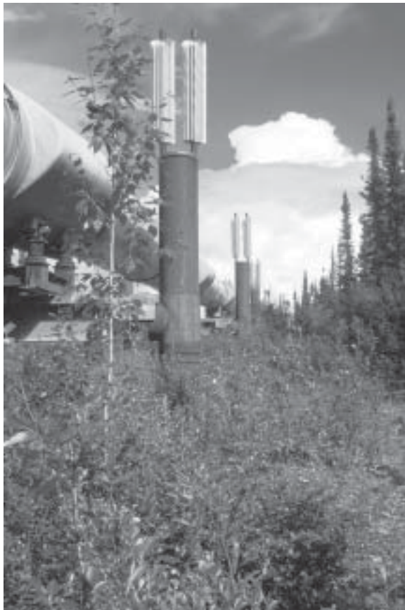
Photo 1. Cottonwood sapling and shrubs invaded around elevated pipeline in Dietrich Valley (23 July 1997). Vegetation development such as this occurs throughout TAPS corridor in the boreal zone. Alyeska Pipeline Service Company periodically cuts this growth either mechanically or by hand.
